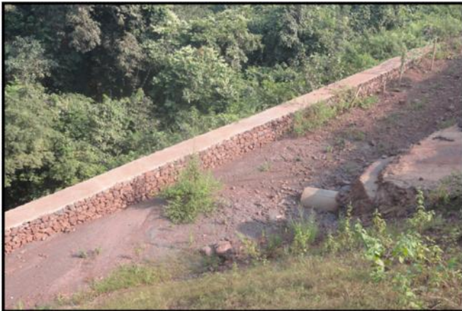
Photo 8– Check Weirs to check Run-off
