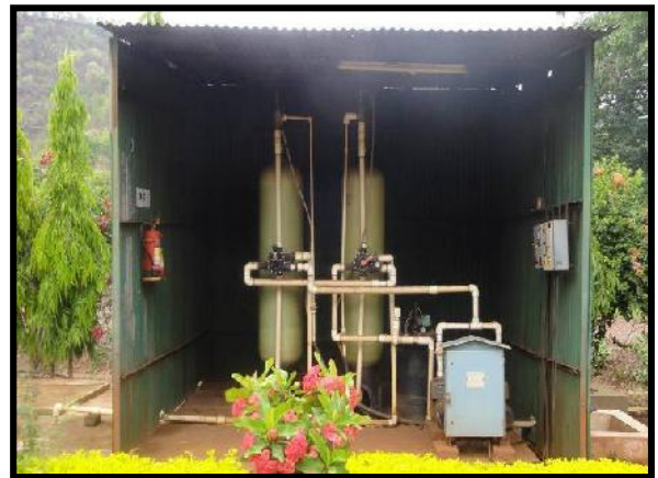
Photo-9 : Showing the STP for treatment of domestic waste water
